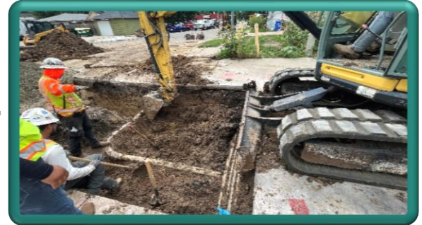
Removal of concrete pavement and excavation within Sweetheart Alley, west of Washington Avenue
