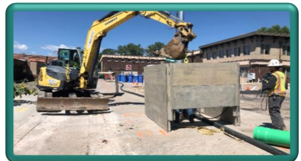
Preparing trench box for placement within Sweetheart Alley, west of Washington Avenue
