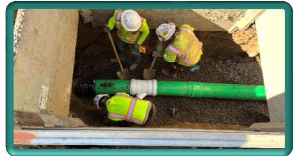
New 12" wastewater main and service connection in Sweetheart Alley, west of Washington Avenue
