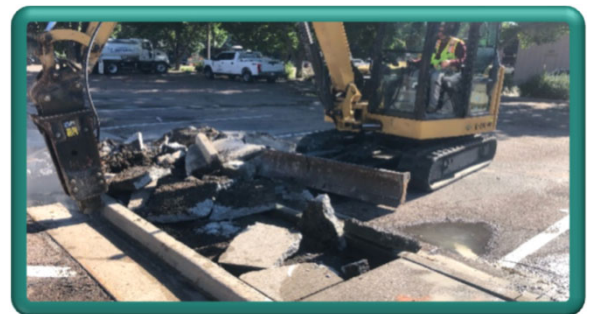
Modifications to the City of Loveland Development Center parking to keep operational during construction
