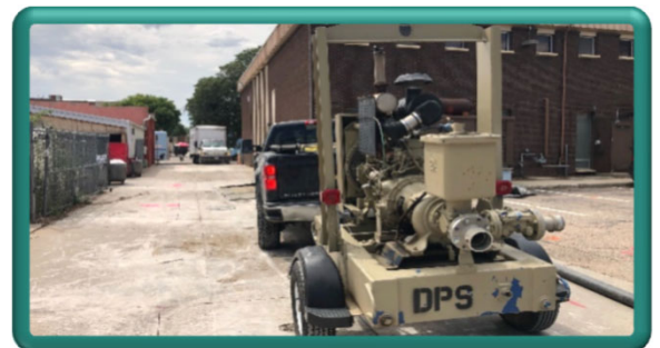
Bypass pumping equipment delivered to job site
