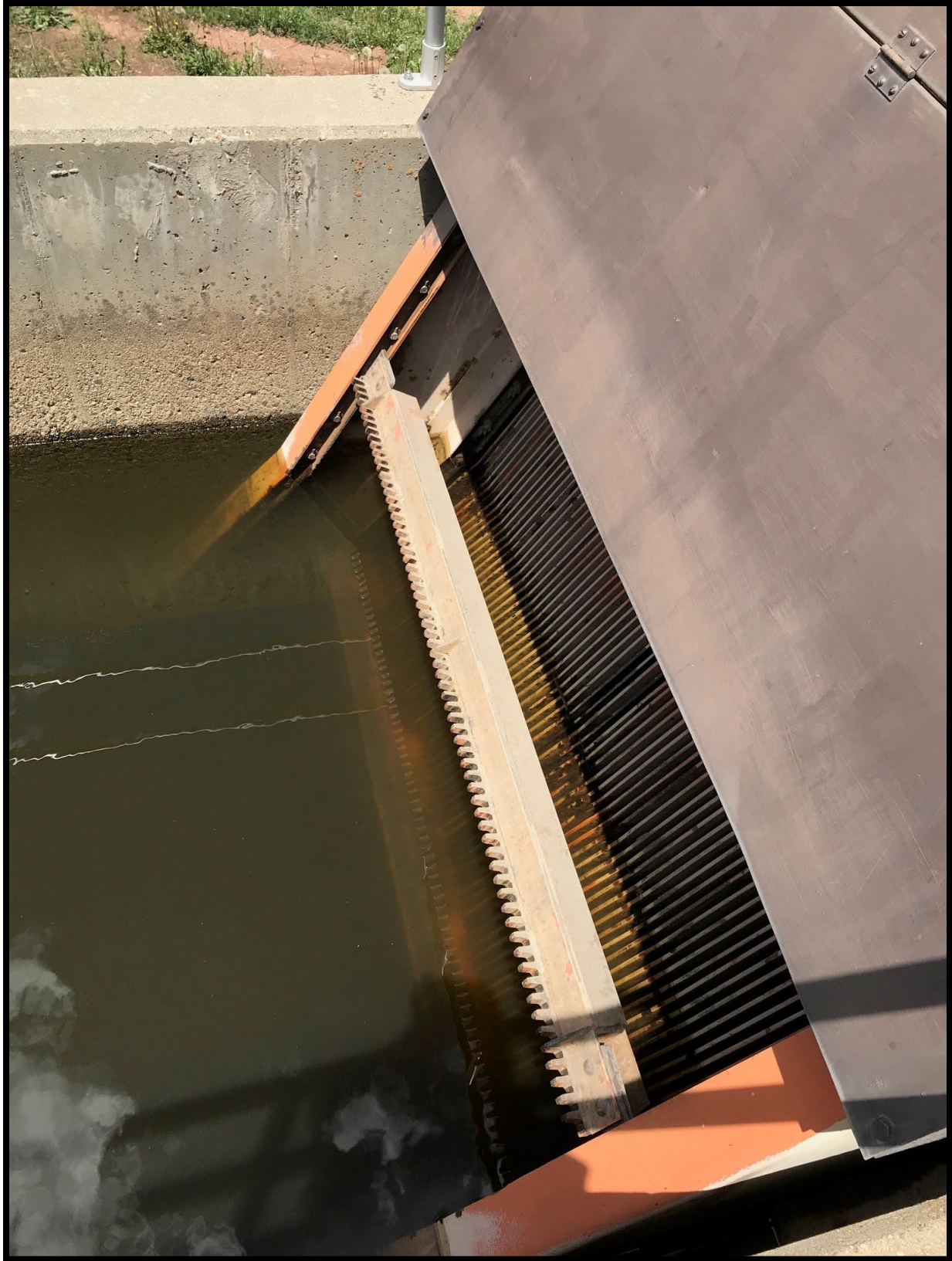
Figure 8. Loveland Water and Power Big Thompson River intake structure.
