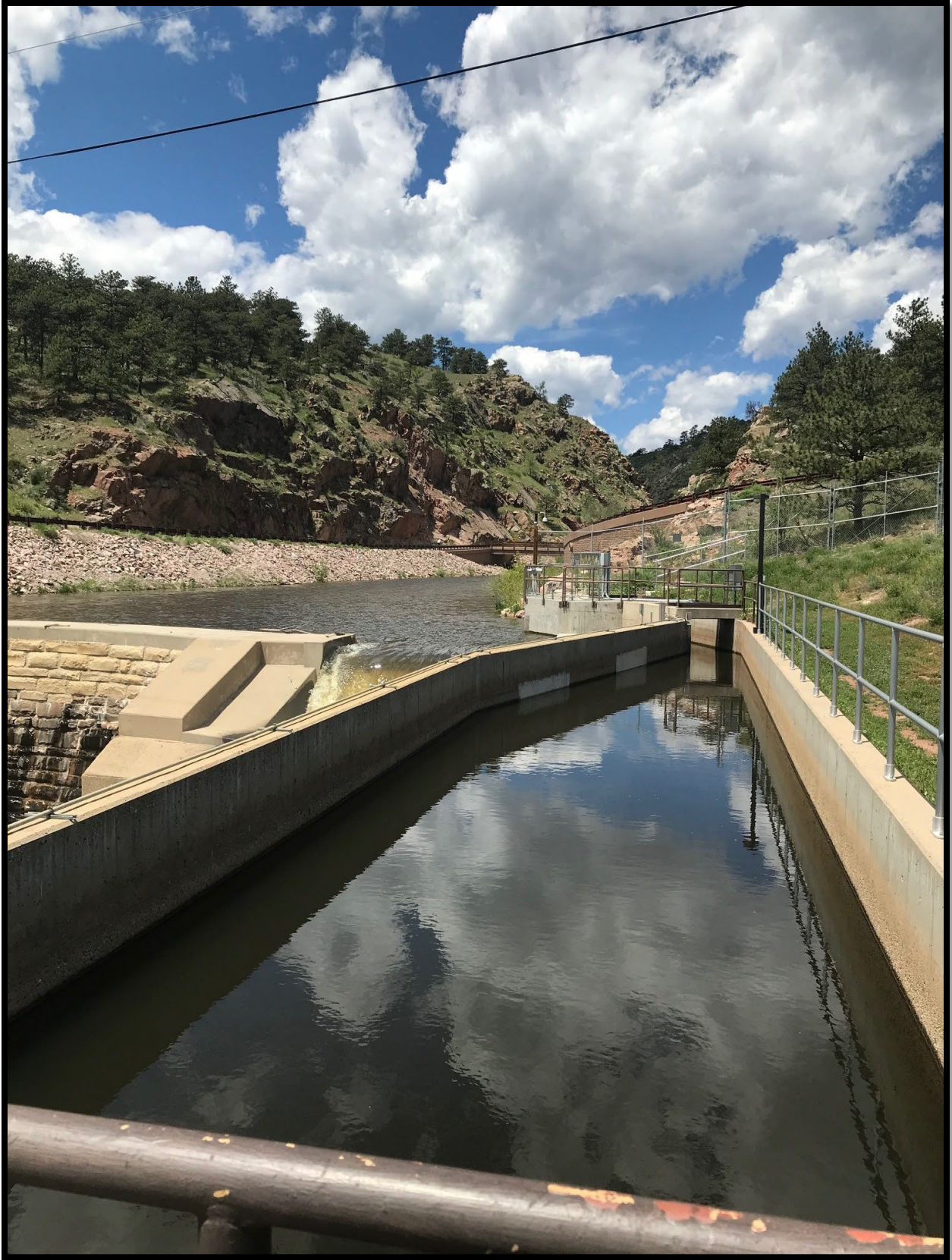
Figure 9. Loveland Water and Power Big Thompson River intake structure.
