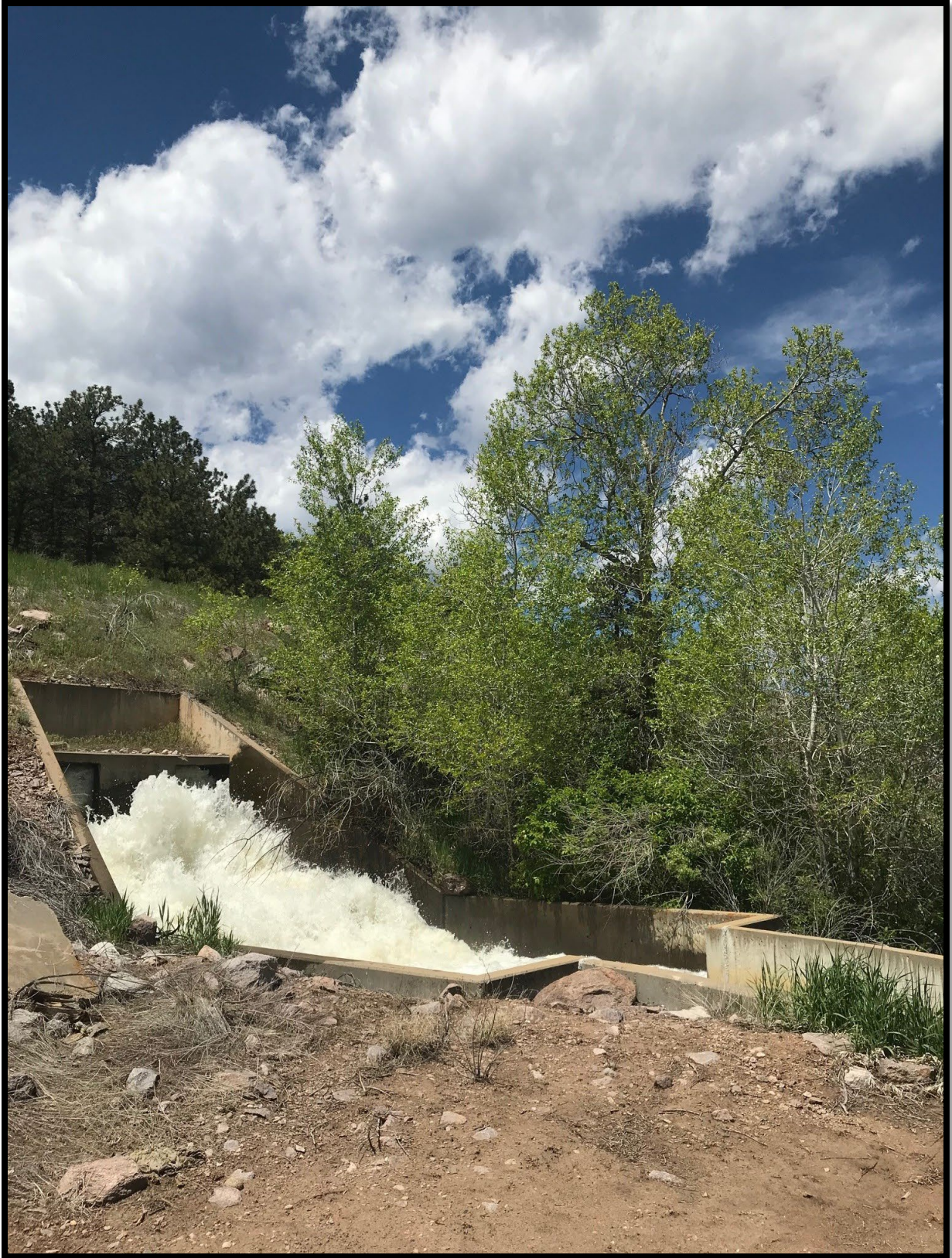
Figure 10. Loveland Water and Power Hansen Feeder Canal intake structure.
