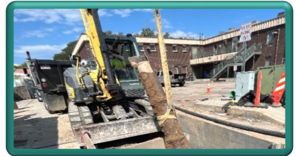
Removal of old 10" clay wastewater pipe for replacement with new 12" PVC pipe
