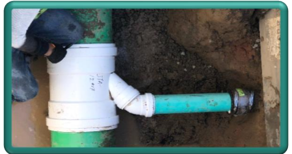
Re-establishment of private wastewater service to the new main in Sweetheart Alley
