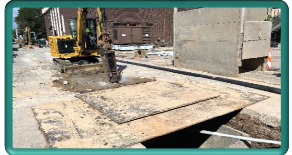
Removal of concrete pavement within Sweetheart Alley for continued excavation of wastewater main trench
