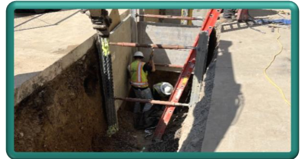
Trench excavation and shoring - Excavations down to existing wastewater pipe are approximately 10' deep.
