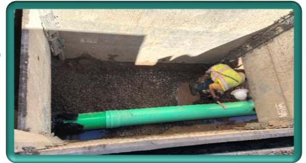
Installation of new wastewater pipe within Sweetheart Alley, between Washington Ave & Jefferson Ave
