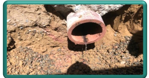
Existing service lateral prior to reconnection. The majority of the existing wastewater main and private service pipes are made of clay.
