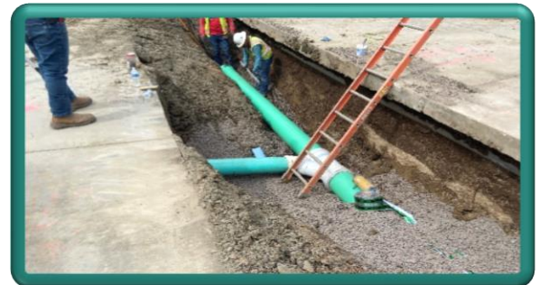
Continuation of new storm drain pipe installation, looking west down the Sweetheart Alley
