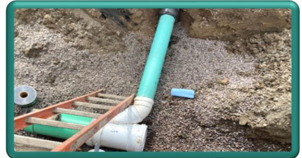
Reconnection of existing roof drain lateral to the public storm drainage system
