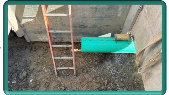
Continuation of storm drain pipe replacement in alley between Washington and Jefferson Avenues
