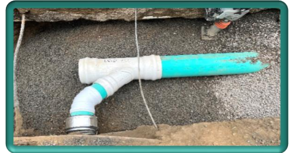
Storm drain installation and roof drain lateral reconnection in alley, west of Jefferson Avenue
