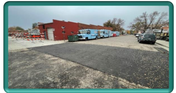
Road closure signs have been pulled and Jefferson Avenue is open following placement of new asphalt
