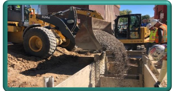
Placement of backfill material atop new wastewater pipe installation in Jefferson Avenue
