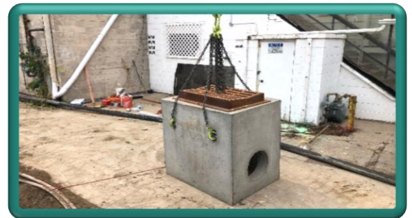
A storm drain inlet being prepared for placement in the alley between Jefferson and Lincoln Avenues
