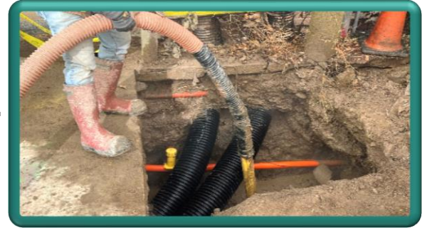
Hydroexcavation uses high pressure water hoses and vacuums to excavate around vulnerable utilities that may be damaged by heavier equipment
