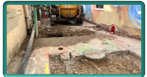
Removal of concrete pavement in the alley between Jefferson and Lincoln Avenues
