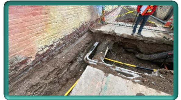
The narrow alley and multitude of existing utilities creates challenges for excavation and requires patience and caution
