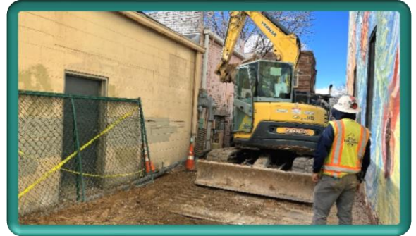
The last section of pipe installation between Jefferson Ave and Lincoln Ave present the most restrictive working conditions for our contractor
