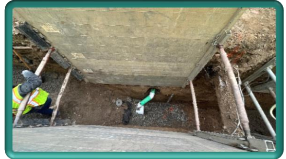
The new wastewater pipe in the alley is approximate 9' deep - the contractor utilizes trench boxes to create an accessible work area for the crew
