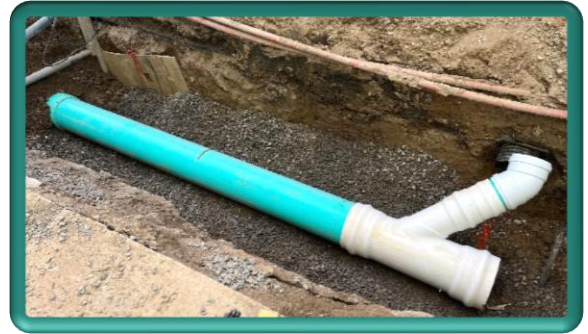
Installation of storm drain pipe and reconnection of a building roof drain to the storm drain collection system
