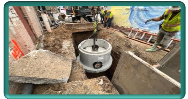
Installation of final sanitary sewer manhole in the Alley, between Jefferson and Lincoln Avenues
