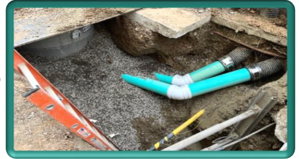
Connection of storm drain into the last manhole in the Alley, between Jefferson and Lincoln Avenues
