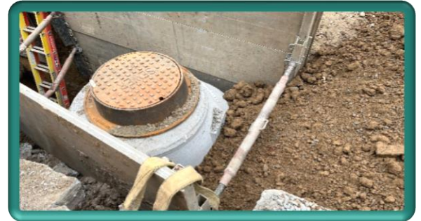
Completed installation of final sanitary sewer manhole, prior to backfill and paving
