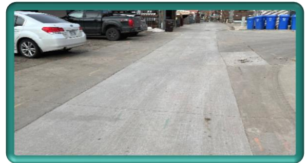
Block A (Washington Avenue to Jefferson Avenue) construction complete and re-opened to vehicle access
