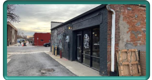
Block B (Jefferson Avenue to Lincoln Avenue) construction complete and re-opened to vehicle access
